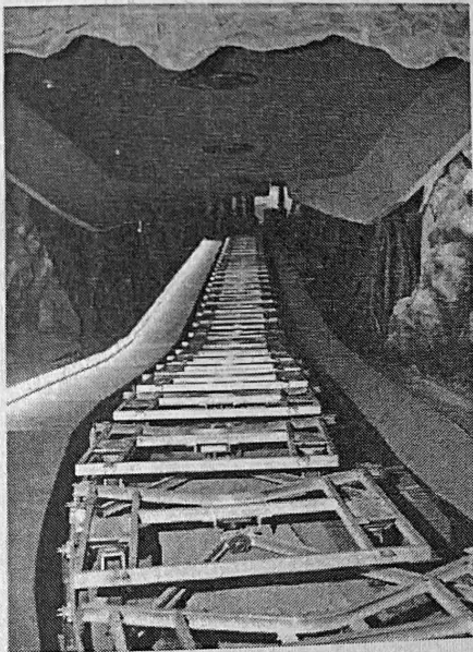
Fig. 3—A service walkway parallels the entire length of the track. This walkway is automatically lighted in case of emergency, as shown in this photograph taken during construction. Cardboard dust shields, used temporarily during the construction period, appear over the continuous center opening of the track.
